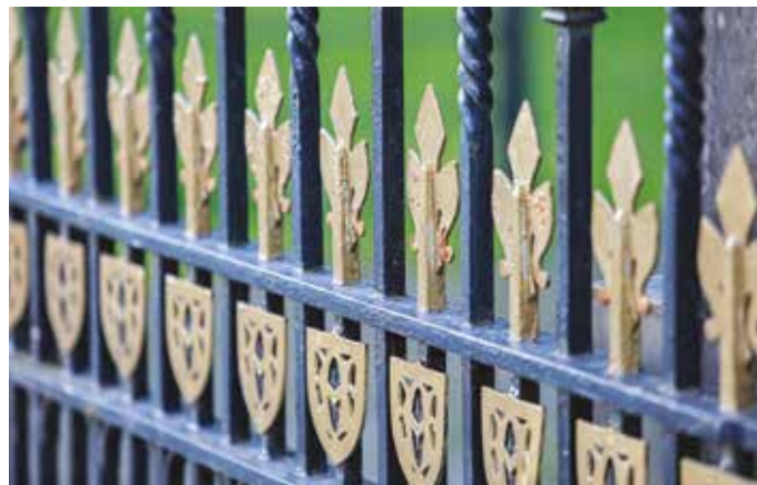
Cast iron entrance gate at Muckcross House, Killarney (image by Valerie O'Sullivan)
